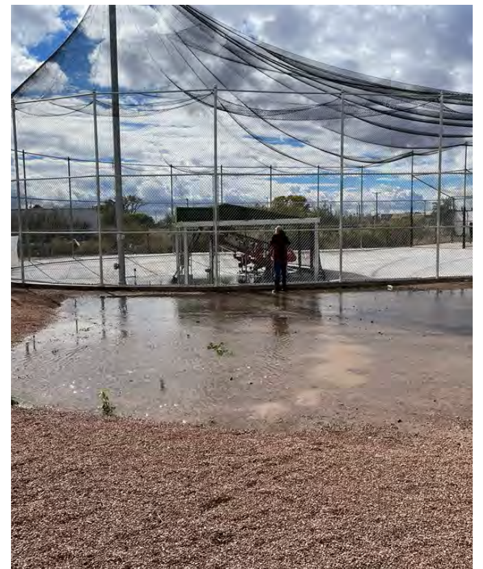
Flooding at Inclusive Park and the Starmax batting cage. GSI practices can re-purpose stormwater to irrigate plants, creating a more vibrant and beautiful city while helping to address flooding problems.
