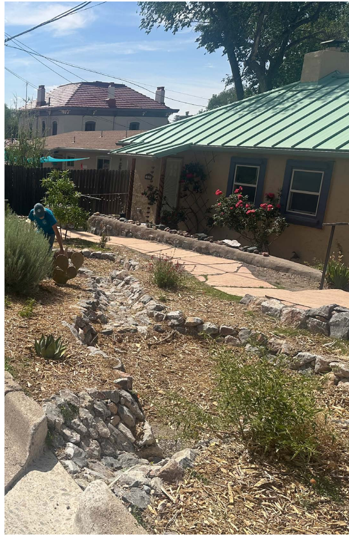
A green stormwater infrastructure (GSI) feature with curb cut, bioswale and basins in Silver City constructed by Asher Gelbart, Green Energy Now, that will harvest rainwater to irrigate the landscape and reduce flooding in streets during storm events.
