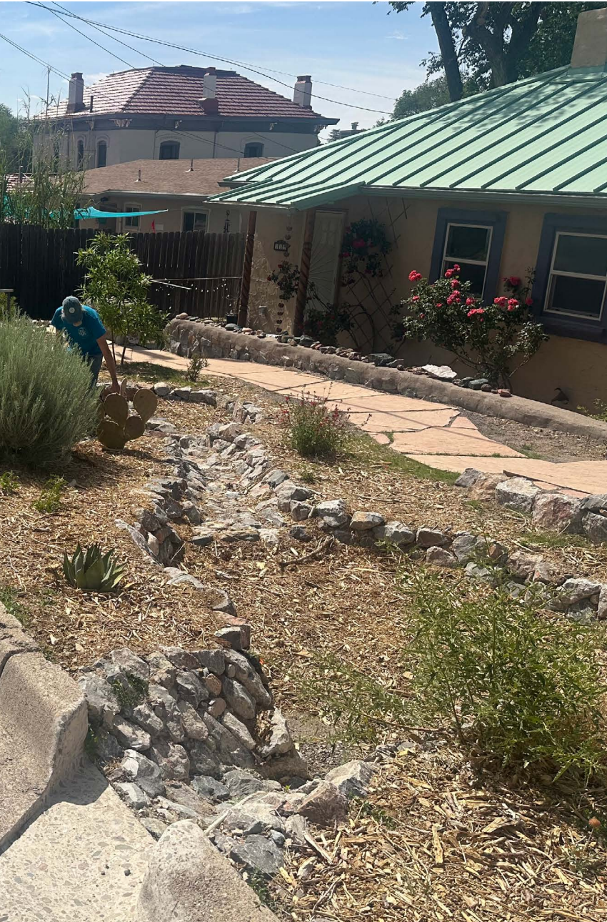
Curb cut, bioswale and basin complex in Silver City constructed by Asher Gelbart, Green Energy Now, that will allow stormwater to irrigate the landscape and reduce flooding in streets during storm events.
